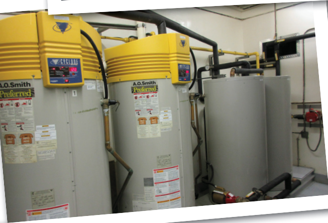
Top to Bottom: Museum (tongs, ice chests, window cards, antique trucks, ice pictures, lunchroom and lockers through doorway); North Star Ice trucks; Domestic hot water heaters (AOSmith 98% efficient cyclone)
